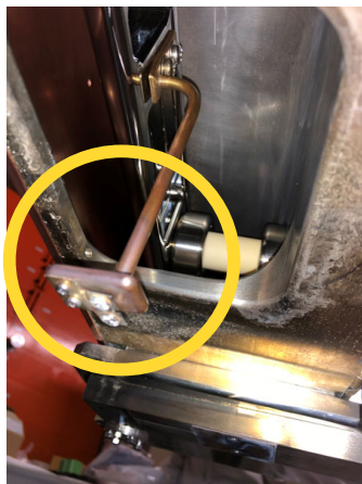
The contact pole is slightly declined and the contact is not sufficient.
